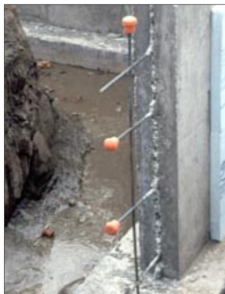
Figure 5. The exposed ends of rebar can cause fatal accidents. OSHA regulations call for rebar ends to be covered with high-visibility protective caps.
