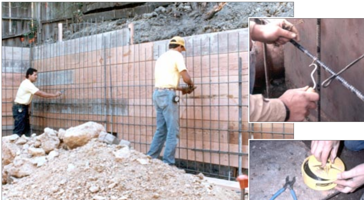
Figure 4. The author ties the rebar at every intersection. Precut wire can be bought in bundles and twisted with a special swiveling tool (top right), but the author's crew prefers to use a pair of spring-loaded linesman's pliers and a roll of wire on a spool (right).
