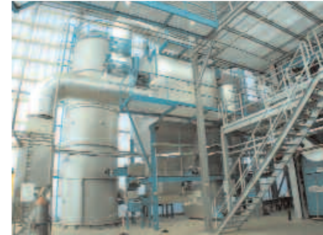
Figure 2: Flue gas cleaning.
