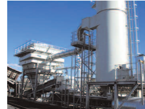
Figure 2: Bio-fuel hopper including dust suction and filtering systems.
