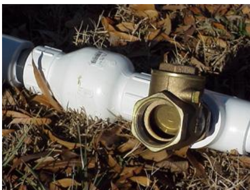
Figure 12. A brass swing check valve. Note the free-swinging flapper in the outlet port. The swing check valve should be placed vertically for best pump performance. Photo credit: W. Bryan Smith, Clemson University.
