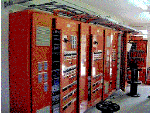
Fig. 29 Electrical Control Panels (Grundfos Pumps, September 2002)
