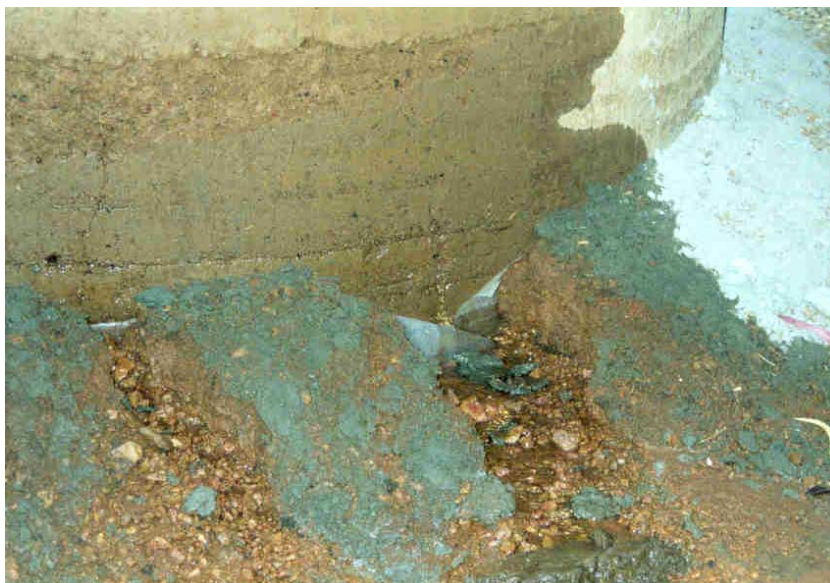
Figure 7.11 Failure of RE2 through 'piping' – this figure shows the leakage at the base of the tank and the crack running through the wall
