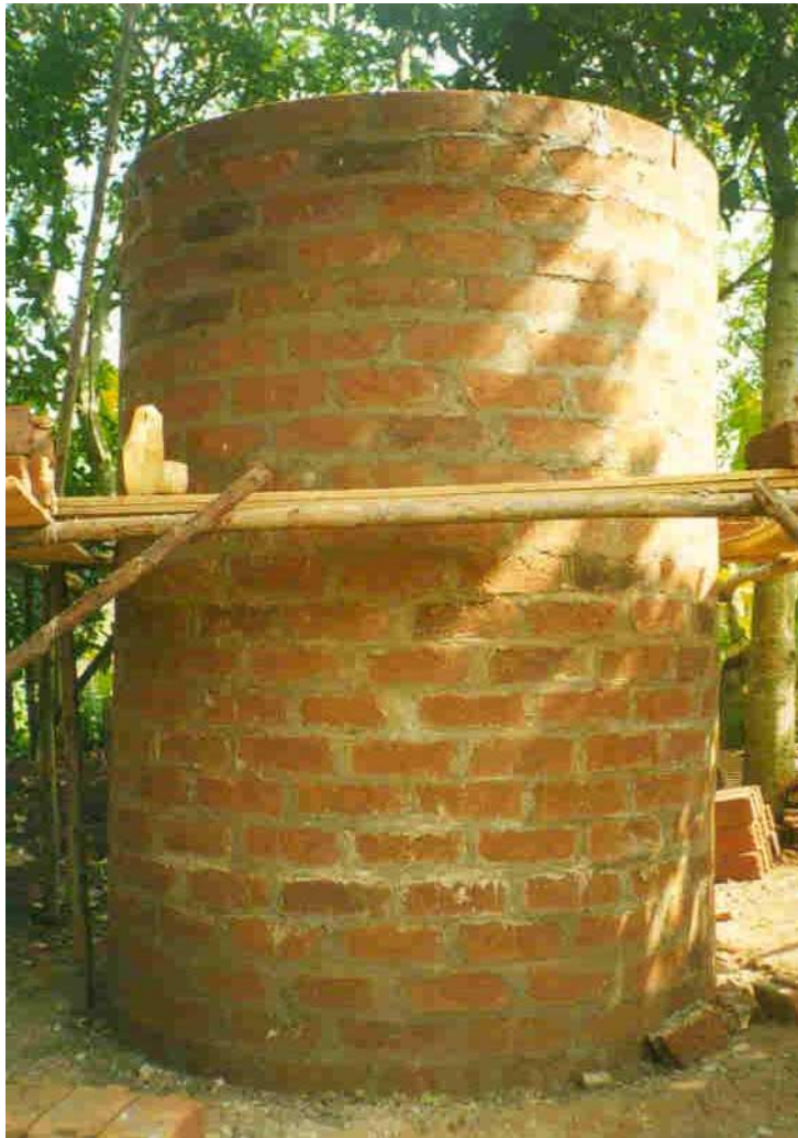
(Figure 6.4 – A SSB tank of 1.67m diameter)
