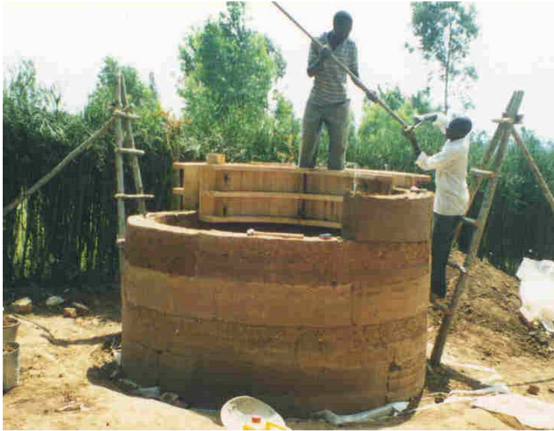
Figure 7.10 The experimental rammed earth tank under construction at Kyera Farm, Mbarara, Uganda.
